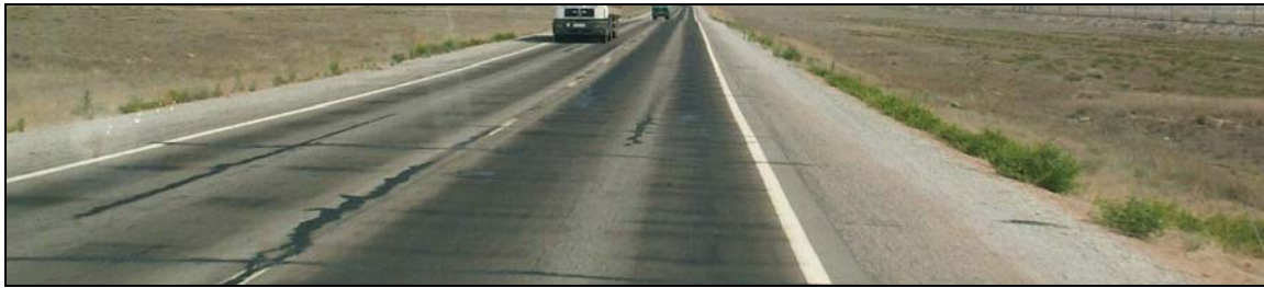
Typical road section showing transverse thermal cracking. The cracks have been sealed during normal maintenance operations. Although the road appears somewhat unsightly considering its age, the roughness of the road has not been significantly affected and traffic moves at high speeds.
