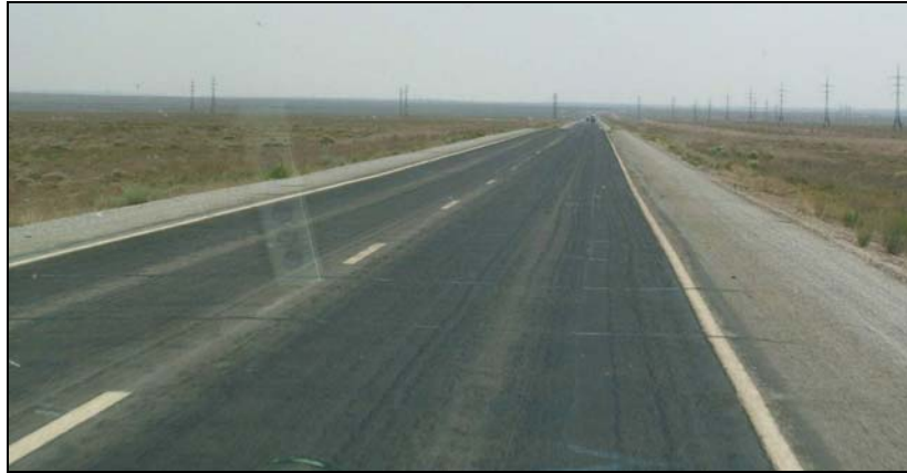
Typical road section performing adequately in carrying high-speed traffic, but showing some transverse cracking.
