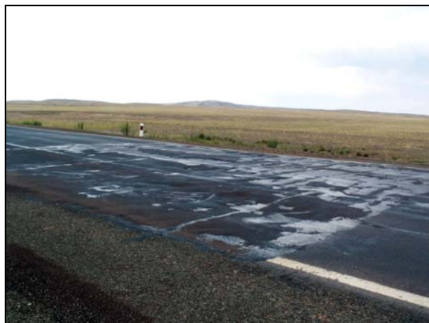
One of the 5–10 localized sections of severe degradation, each of roughly 10–20 m in length.
