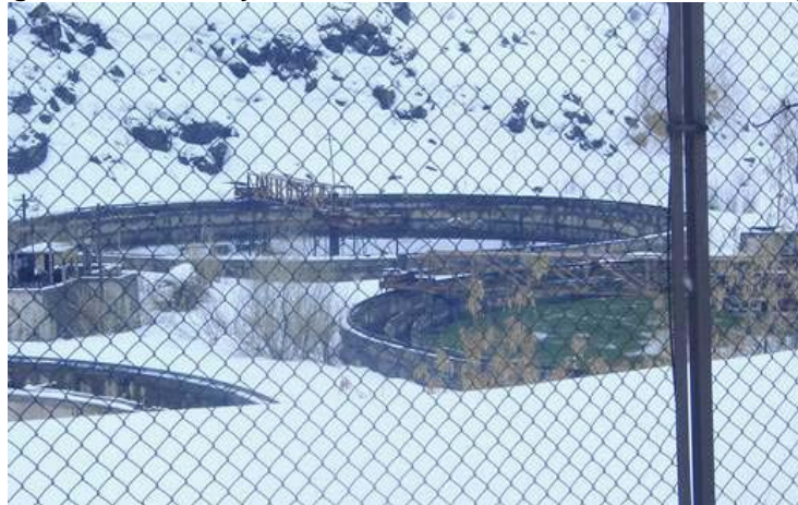
Figure 2.7 Secondary sedimentation tanks, WWTP at Kakhsi village
