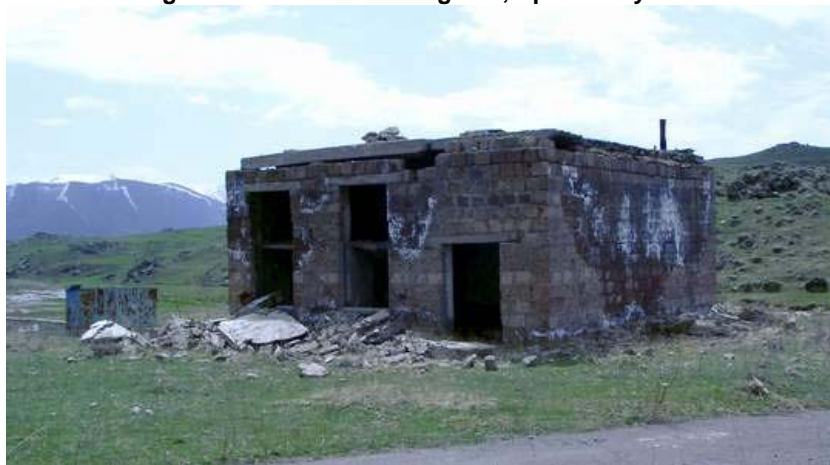
Figure 2.9 The Chlorinating unit, Aparan city
