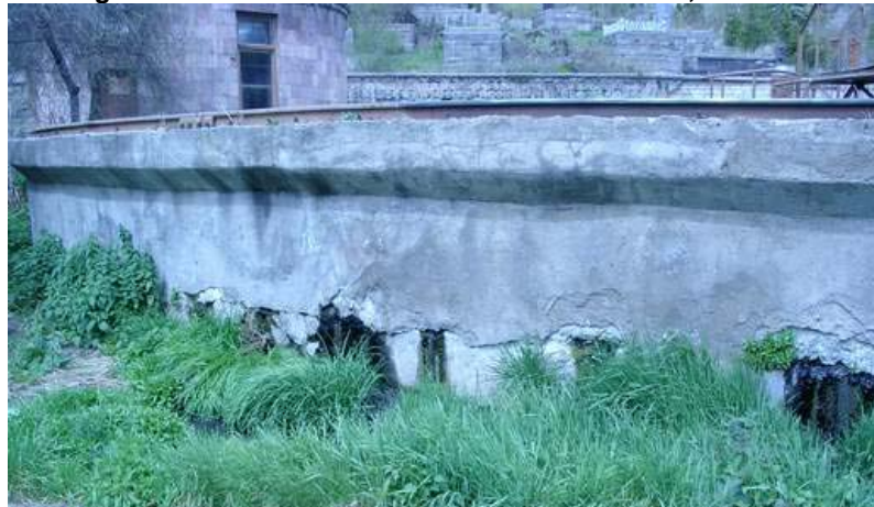
Figure 2.16 Sedimentation reservoir's seal failure, Vanadzor
