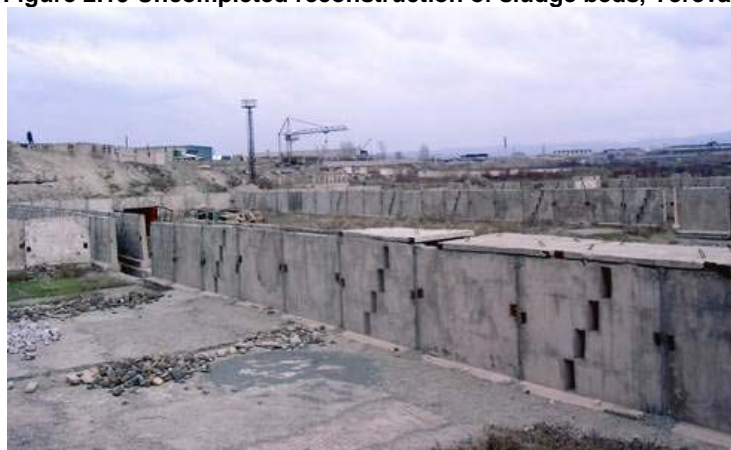
Figure 2.19 Uncompleted reconstruction of sludge beds, Yerevan
