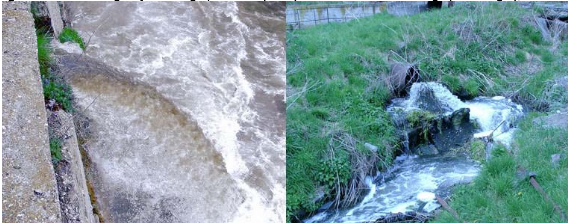
Figure 2.15 The emergency discharge (on the left) compared to effluents discharge (on the right), Vanadzor
