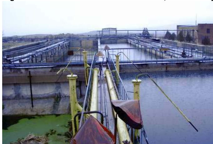
Figure 2.13 The combined treatment facilities, Ashtarak city
