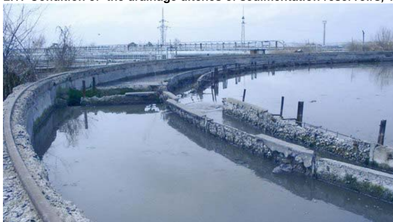
Figure 2.17 Condition of the drainage ditches of sedimentation reservoirs, Yerevan.
