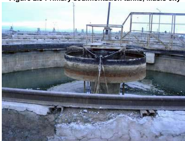
Figure 2.5 Primary sedimentation tanks, Masis city
