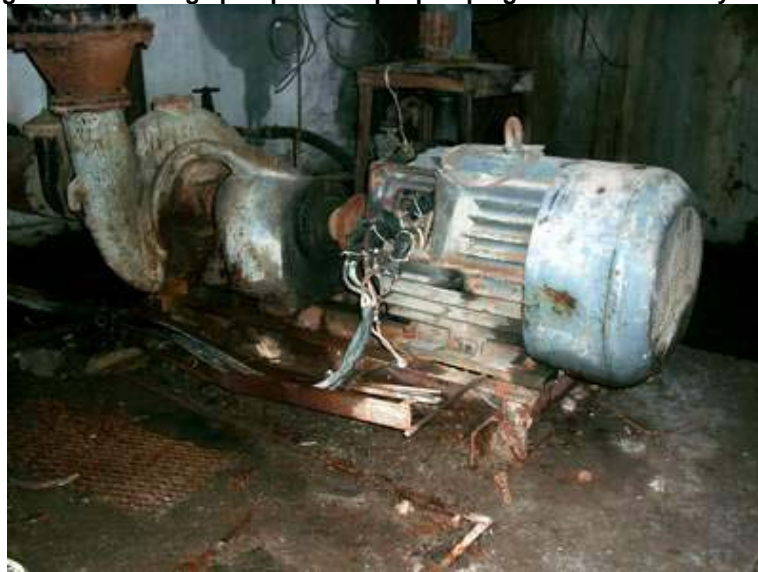
Figure 2.1 Sewerage pump. Municipal pumping station. Masis city.
