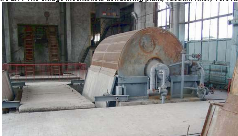
Figure 2.11 The sludge mechanical dewatering plant, vacuum-filter, Yerevan city
