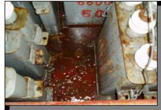
[Improper storage of PCB waste]
