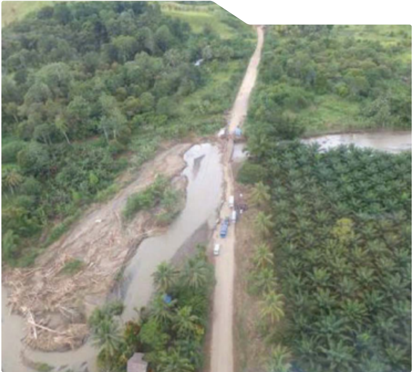
Damaged bridge on the Ramu Highway. Wash outs of bridges and culverts are a common along PNG's roads, meaning particular attention needs to be paid to drainage and water crossings.
