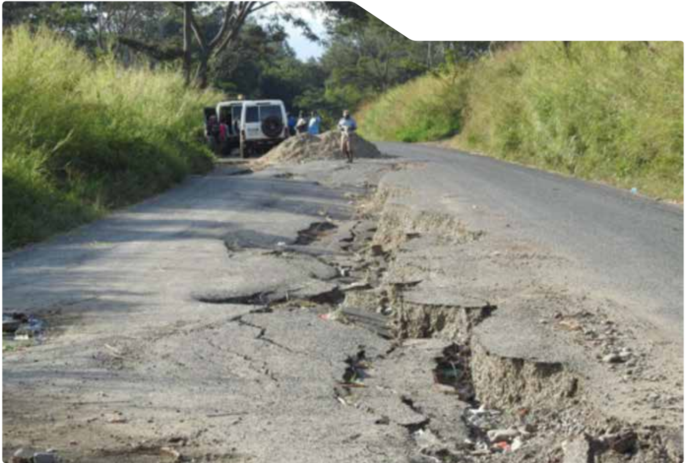
Highlands Highway near Goroka. Much of the national road network is in a poor condition. Sections of road like this one are not uncommon. Photo: Matthew Dornan.
