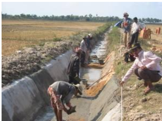
Construction of a canal through the collaboration between municipalities and water users' association
