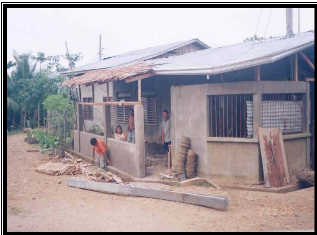
Residents of a resettlement site in Pagadian City rebuild their homes into sturdier and durable materials.
