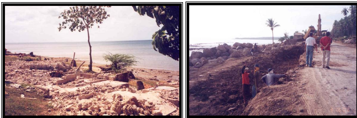
Structures along the Mulanay coastline were demolished to give way for the road improvement works of the Sixth Road Project.
