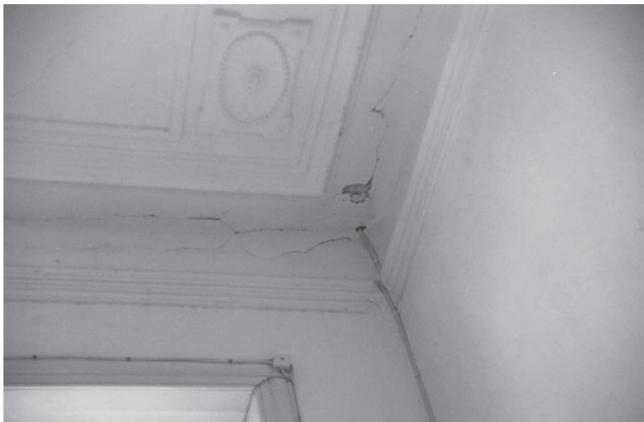
Figure 8.5. Cracking of stucco ceiling at Horta (Coronel Silva Leal) school
