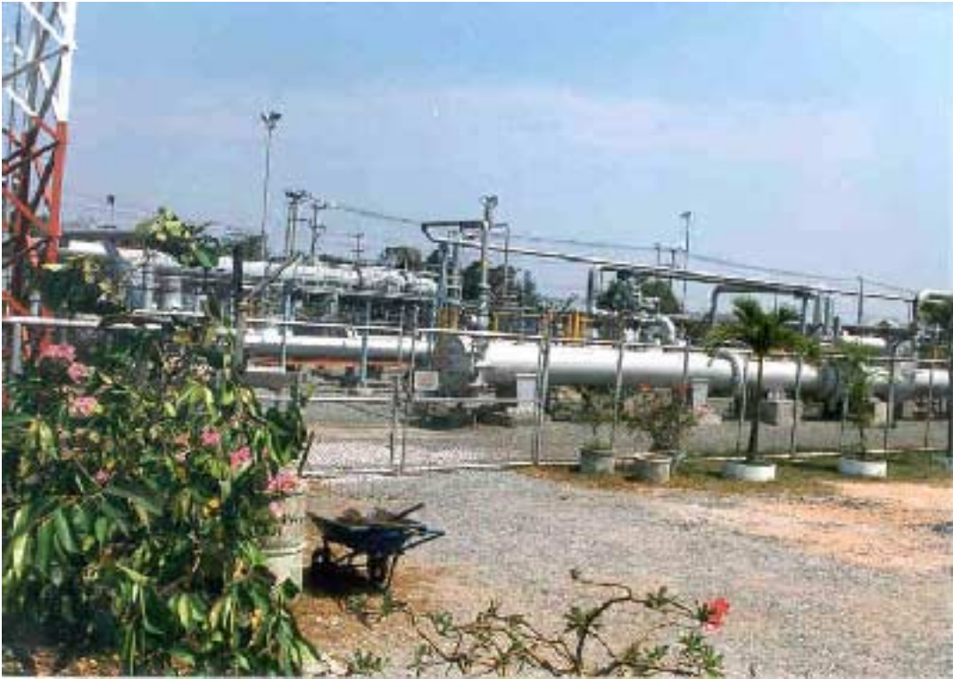
Photo 1: End of onshore pipelines where gas flow, pressure and temperature are monitored and data are electronically sent to the supervisory control and data acquisition (SCADA) control center.
