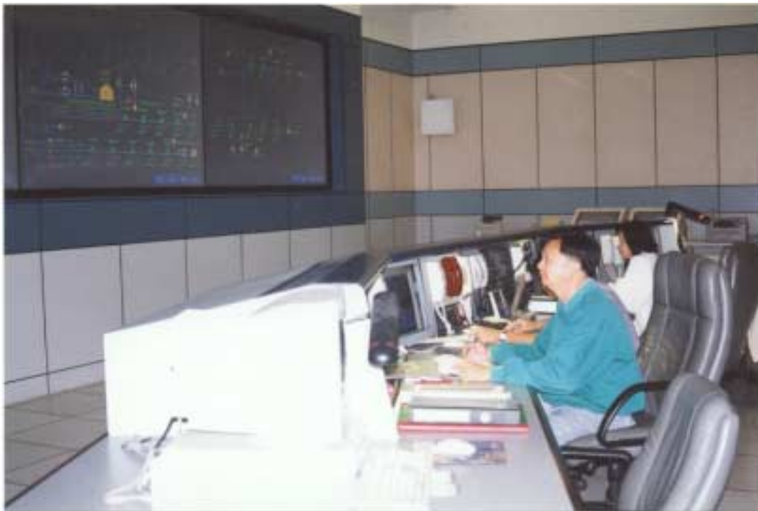
Photo 2: SCADA control center.
